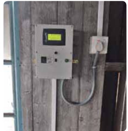
Temperature Controlling System
