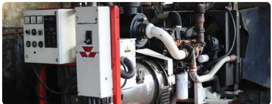
Hydro-Power Plant – Bambrakelley Estate
